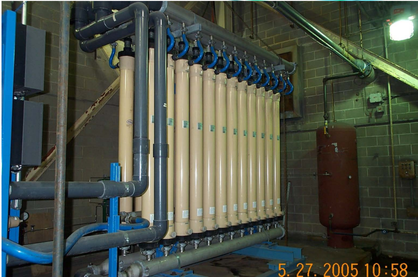
Microfilter pressure vessel skid. Photo by Brad Buecker.
